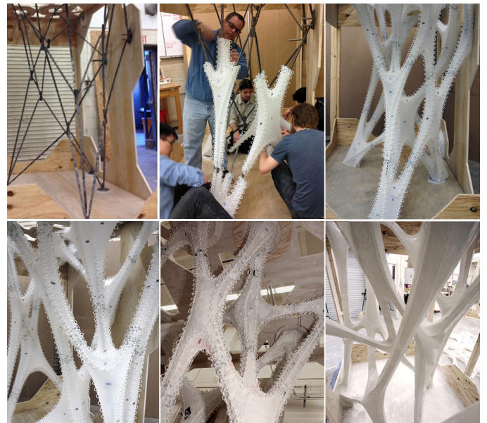
8 Top: Plastic Formwork Assembly Process—(from left) Assembled steel frame, plastic formwork being wrapped around steel frame, and fully assembled plastic formwork. Bottom: Casting Process. (from left) Assembled polypropylene formwork, formwork after casting, unwrapped concrete (Bell 2013).
